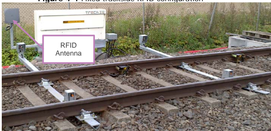
Figure 4-1 Fixed trackside RFID configuration
