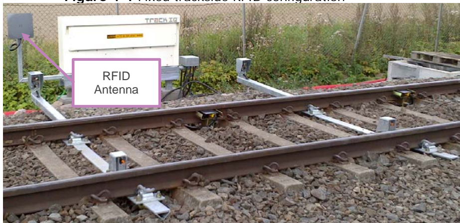
Figure 4-1 Fixed trackside RFID configuration
